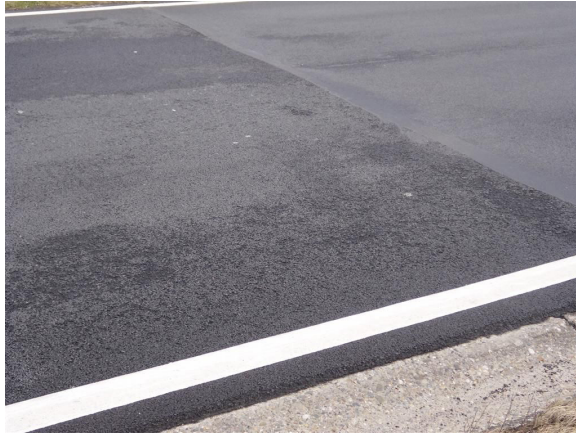
Figure 3: Heavy raveling of a thin surface layer
